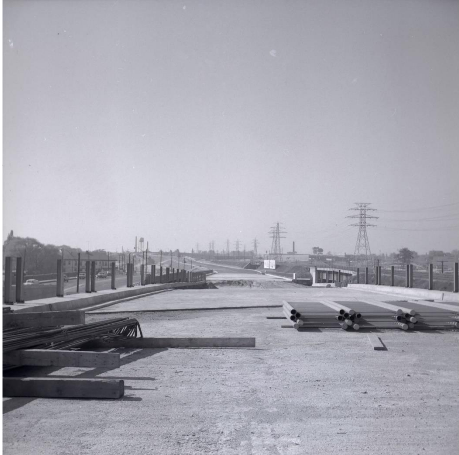
Figure 34: Photograph showing the Former Queen Street Bridge (Mile 5.15) in the right of the photograph (Salmon 1957d).
