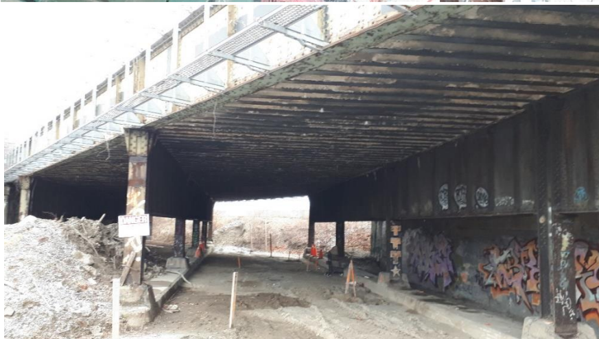
Plate 89: Detail of view under the bridge of the former alignment of Queen Street.
