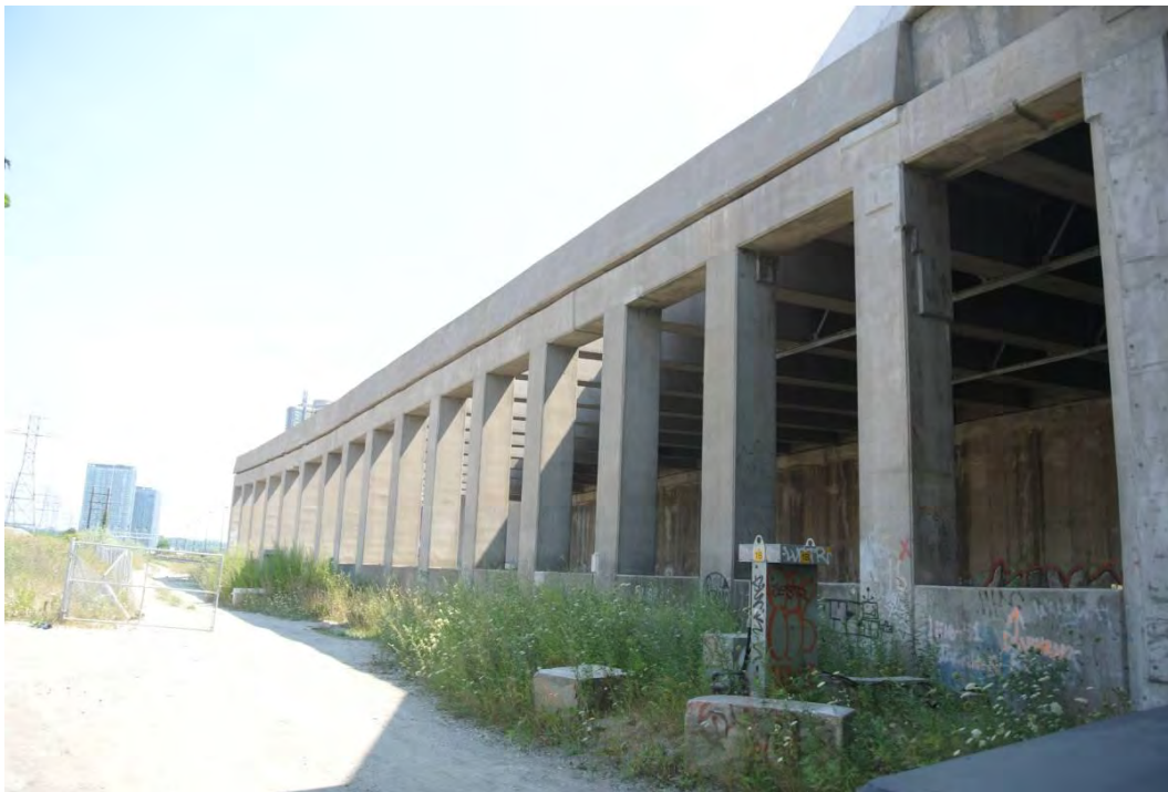
Figure 24: View of the concrete columns extending east from the single pier, looking east.
