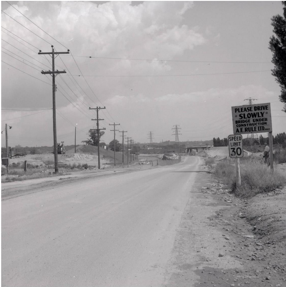
Figure 31: Photograph showing the Former Queen Street Bridge (Mile 5.15) in the distance (Salmon 1956a).
