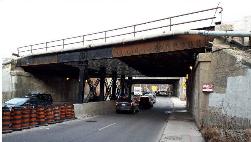
Plate 15: View of eastern abutment and concrete sidewalk along Parkside Drive, looking northwest
