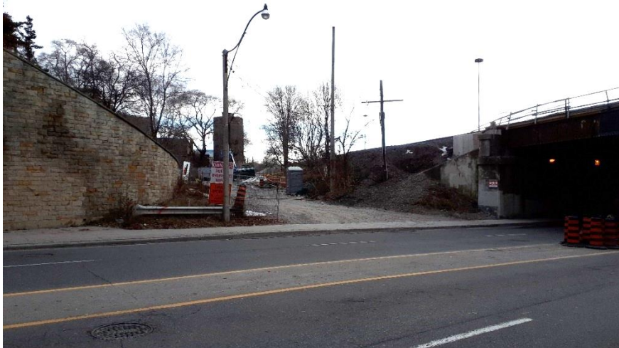
Plate 24: View of construction staging area north of the bridge on the eastern side, looking southeast.
