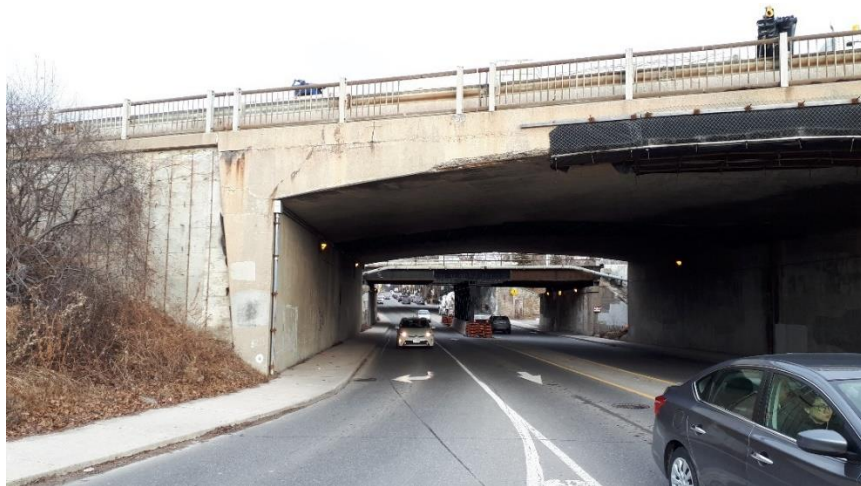
Plate 17: View of Gardiner Expressway bridge south of the Parkside Drive Bridge (Mile 3.89), looking north.
