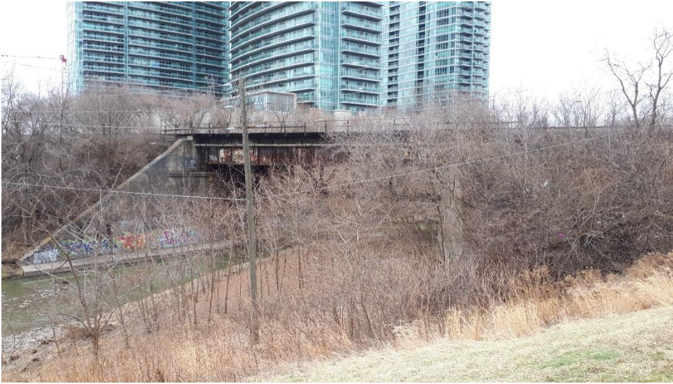
Plate 98: Vegetation growth adjacent to the bridge.
